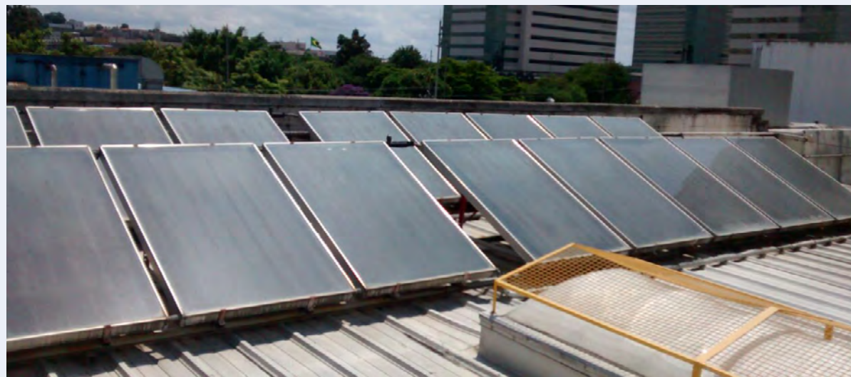
Photo: Solar water heater installed at Baxter's facility in Brazil.
